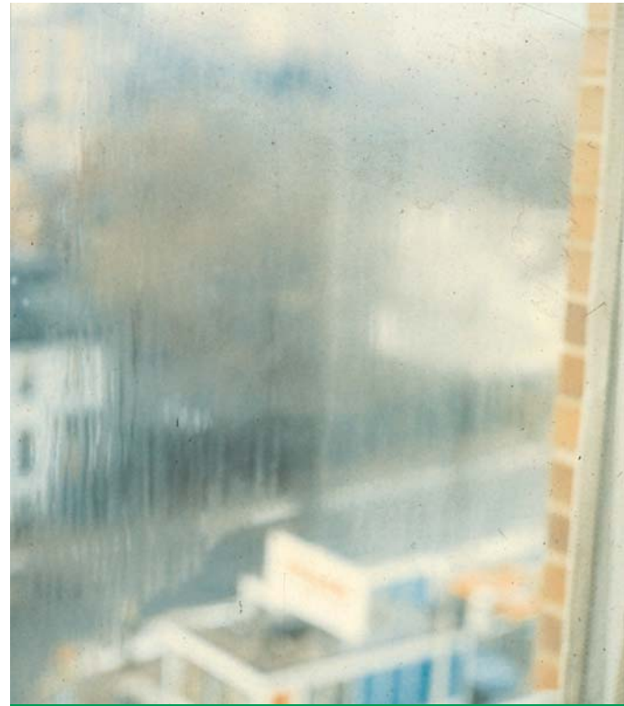
Fig. 13 – Failed IGU Fogged with Condensation
